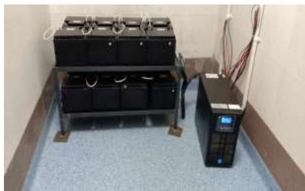
Battery & USP System
